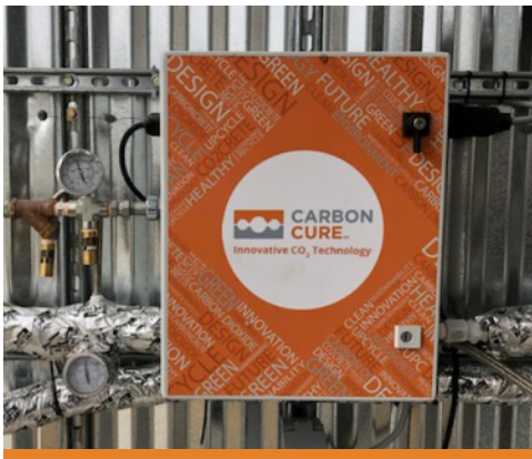
CarbonCure at Ozinga's Miami plant, which became the first CarbonCure system installed in the state of Florida in 2020.
