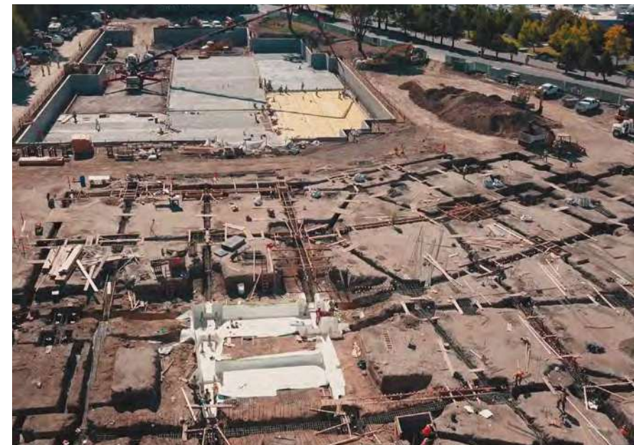
CarbonCure concrete was supplied for the construction of LinkedIn's Middlefield Campus in California.
