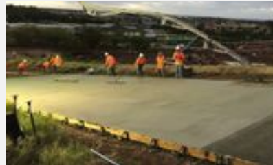
Kapolei, HI – Kapolei Interchange Demo. Concrete Producer: Island Ready-Mix CO 2 Saved: 1,500 lbs
