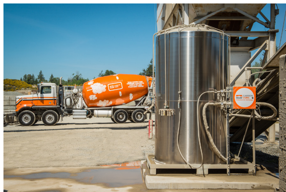
A CarbonCure valve box and CO 2 tank operating at a ready mix plant.
